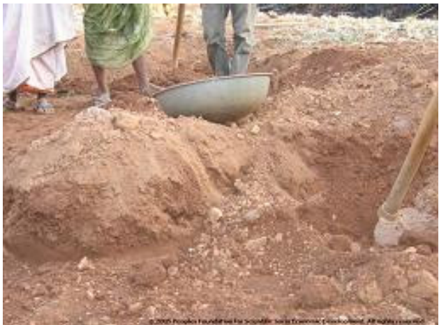
Figure 11: Closer look at the superficial layer which needs removal
